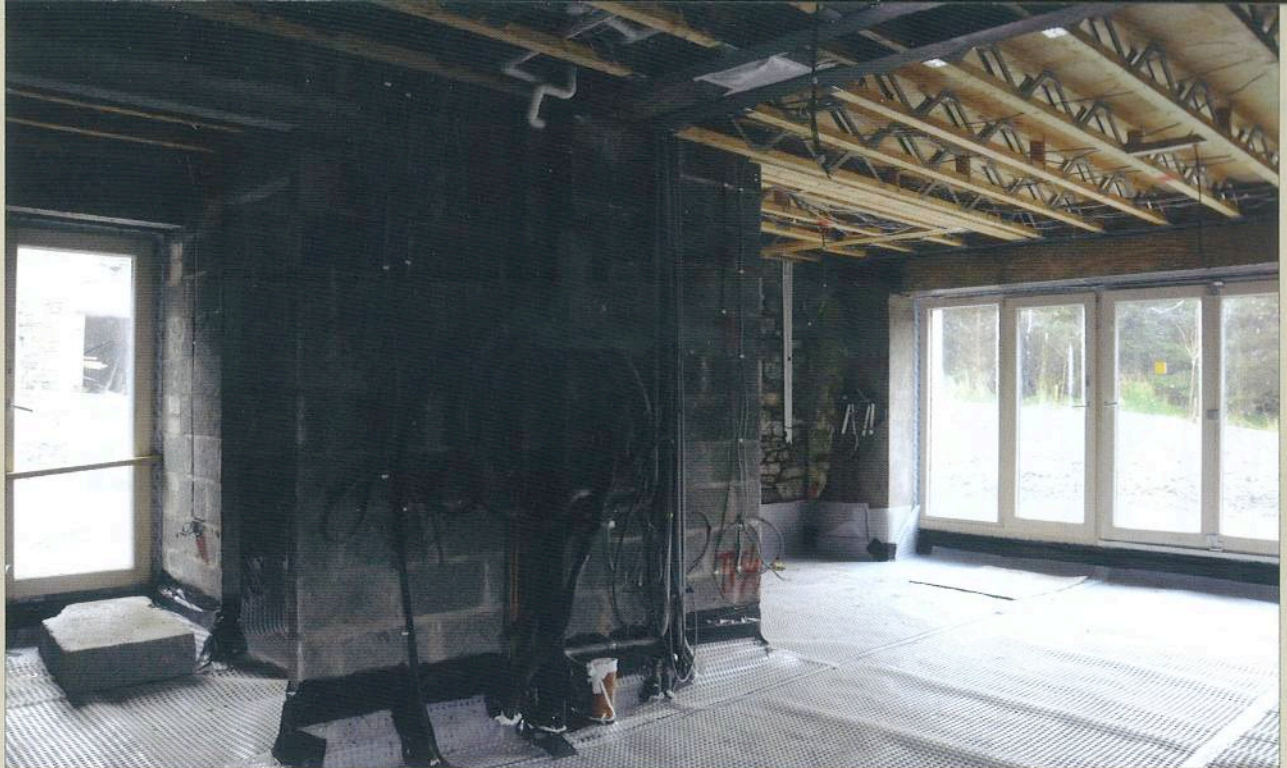
(above) Eco-joists were installed to allow services to travel without interruption to the building fabric; (below) external insulation was fitted to the walls to dramatically increase the thermal performance
